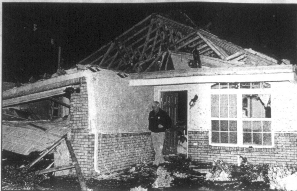
AP Photo Lexington-Fayette Urban County Government Building Inspector Jim Piper walks from a home which was destroyed during a heavy storm Thursday in northwestern Lexington, Ky. At least five recently constructed homes were destroyed.
