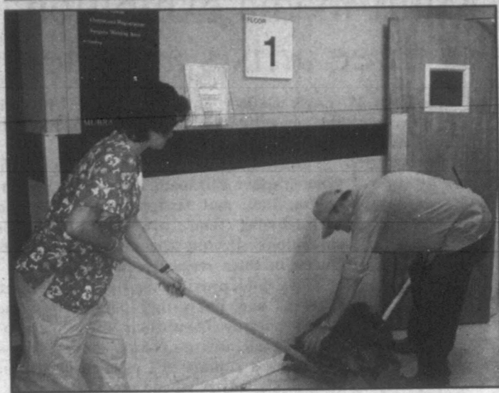
Photo provided Pictured are David Holt and Shannon Kidd, employees in the Maintenance and Environmental Services departments, removing remnants from the carpet pulled from the first floor. MCCH is currently installing new vinyl flooring to replace the carpet on all the patient floors as part of a facility upgrade plan for the hospital.
