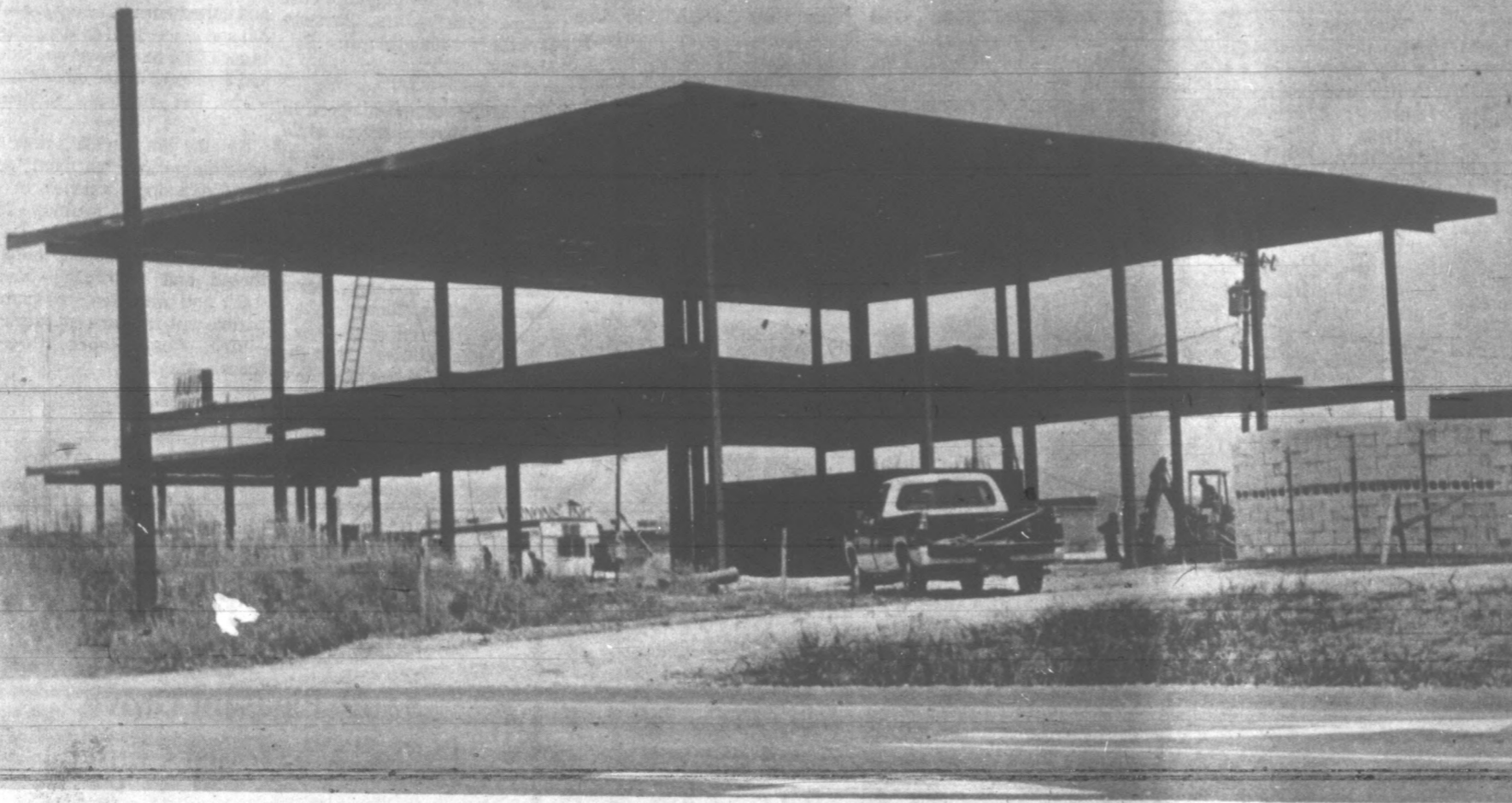
BANK CONSTRUCTION — Construction is only slightly behind schedule, due to weather, on the new University Branch of the Peoples Bank, at 12th and Chest-
