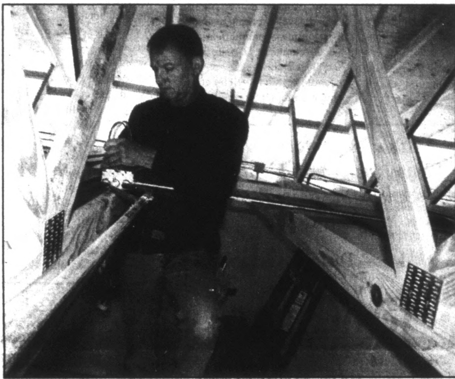
Danny Dunn of Dunn's Electric in Murray works with wiring in the rafters of the new concession building Monday morning at the Bee Creek soccer complex.
