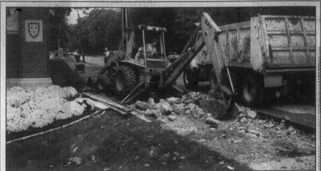
GREG TRAVIS/Ledger & Times TURNING THE CORNER ON PROGRESS: Jimmy Hawthorne uses a backhoe to dig rock at the intersection of Main and 16th streets Tuesday afternoon. The work is part of a renovation of the curb and gutters at the northwest corner, according to Gary Emerine of Emerine Construction of Murray. Also working on the project was Chris Bell in the white truck.
