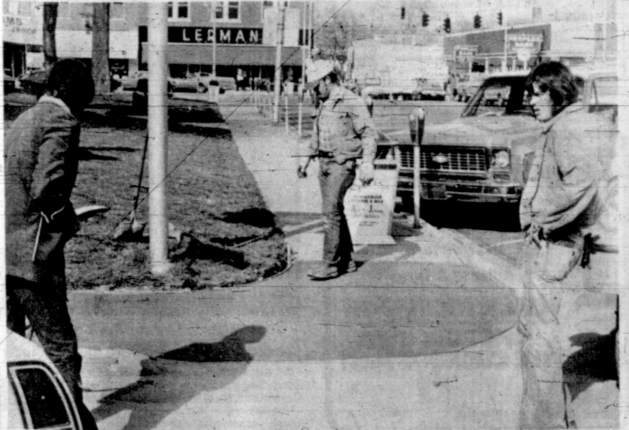
WHEELCHAIR RAMPS — Charlie McKenny and his CETA crew are working this week on wheelchair ramps at the corners of the court square. The ramps will enable wheelchairs to roll from the street to the sidewalk with a minimum of effort.
