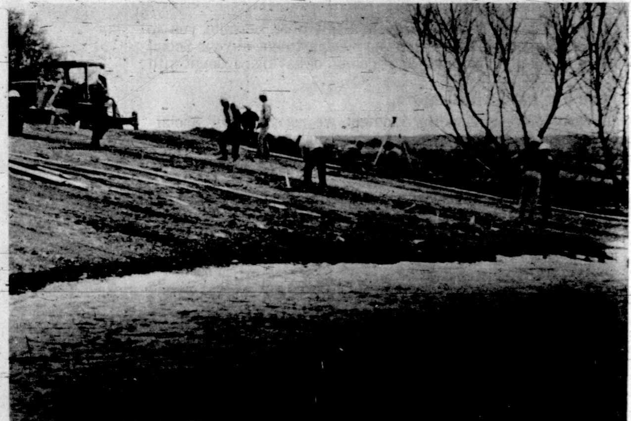
Work is expected to be completed within the next few days on construction of a new boat launching ramp at Fenton Informal Use Area just east of the Egner's Ferry Bridge in Land Between The Lakes, TVA's public outdoor recreation area. The older, smaller ramp presently at the site is being removed and replaced with a new and considerably larger ramp, which will allow three boats to be launched at one time. The new facility is 40 feet wide and 72 feet long and consists of a 6-inch thick concrete slab. TVA employees are completing the work this week.
