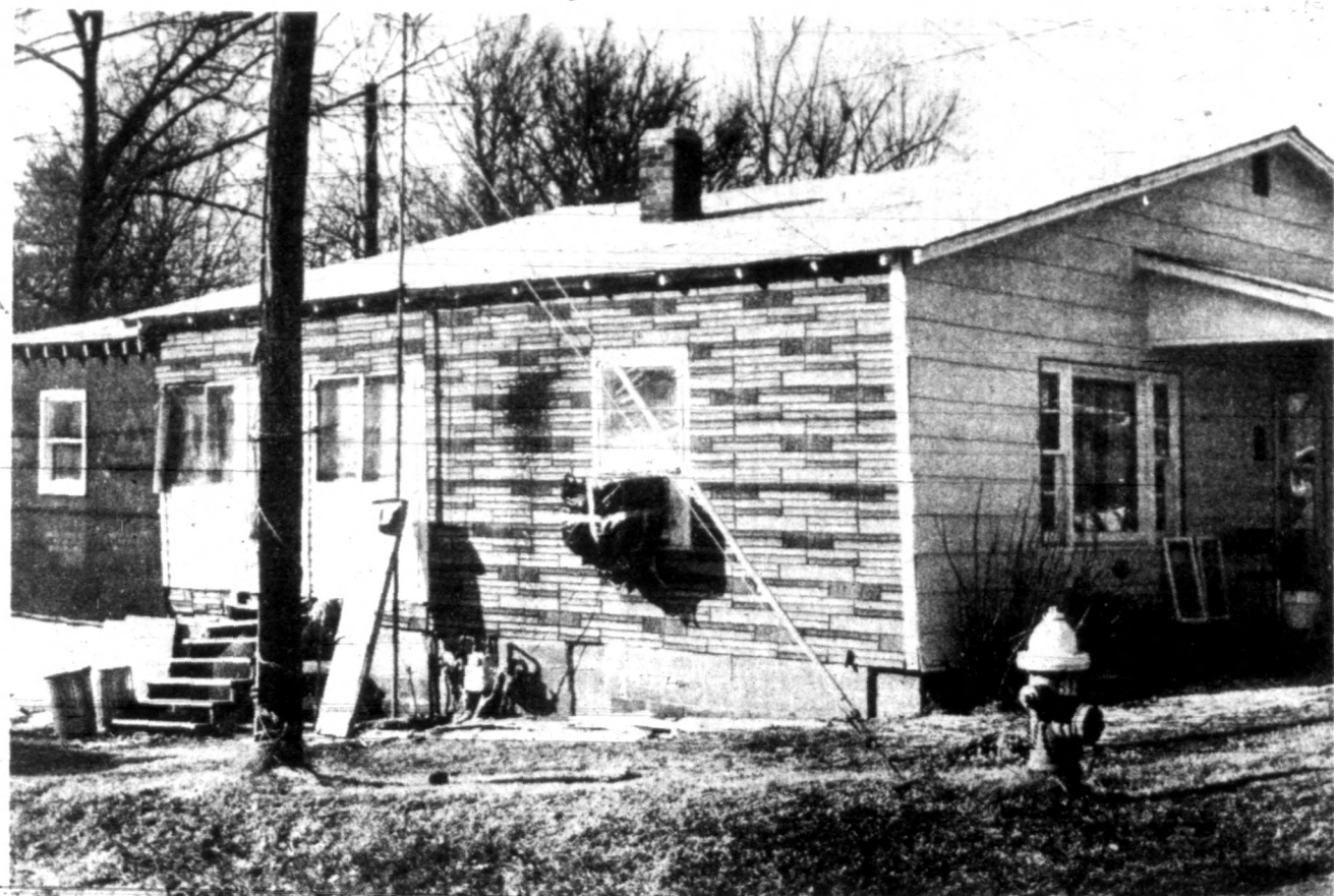
PROJECT UNDERWAY — The community development rehabilitation of houses in the north Douglas Community started near the end of January with this house, 301 Pine Street. The house is receiving aluminum siding and some interior work. The project, funded by a $996,000 grant from the Department of Housing and Urban Development, will upgrade the structural standards of 65 to 70 houses, according to Bobby Henry, director of the local community development agency. The grant primarily is concerned with upgrading house structures. House repairs to be made are determined by the agency and construction company bids are accepted on each house with the contract going to the low bidder, Henry said. Area water lines also will be repaired with the funds. A $10,000 limit has been set for each house but Henry said the figure could be adjusted when necessary. Henry said a greenery area along 2nd Street is being discussed as a joint-project with the Tappan Co. A pre-application for the grant was made in January 1979 and the application was filed in May 1979, Henry said. HUD approved it in October, Henry added. The community development agency will seek another grant when the present one expires in September 1981, Henry said. The second grant would go toward curbs, gutters and road repair, he added.
