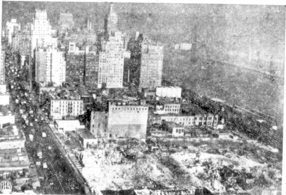
WORK BEGINS ON WORLD CAPITAL —Buildings are being torn down on the little strip of midtown Manhattan, New York, which some day will be the permanent home of the United Nations. This view shows the area involved, five blocks along the East River. At upper right is the Queensboro Bridge.
