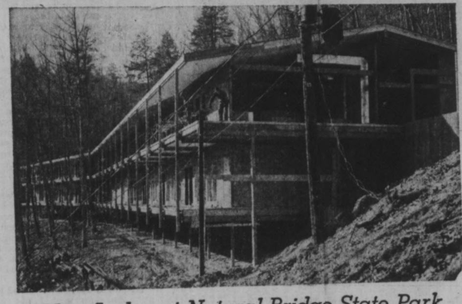
New Lodge at Natural Bridge State Park THIS 24-ROOM LODGE under construction at Natural Bridge State Park, near Slade, is to be completed in time for the 1964 season opening. Cost of the project, including a lobby, lounge, and a 200-capacity dining room, is $639,400. Lane, White and Congleton of Lexington is the contractor. This building, replacing old Hemlock Lodge, makes a total of eight new lodges and room additions to two others in Kentucky's State Parks system in two years. A new lodge also is under construction at Buckhorn Lake State Park, near Hazard.
