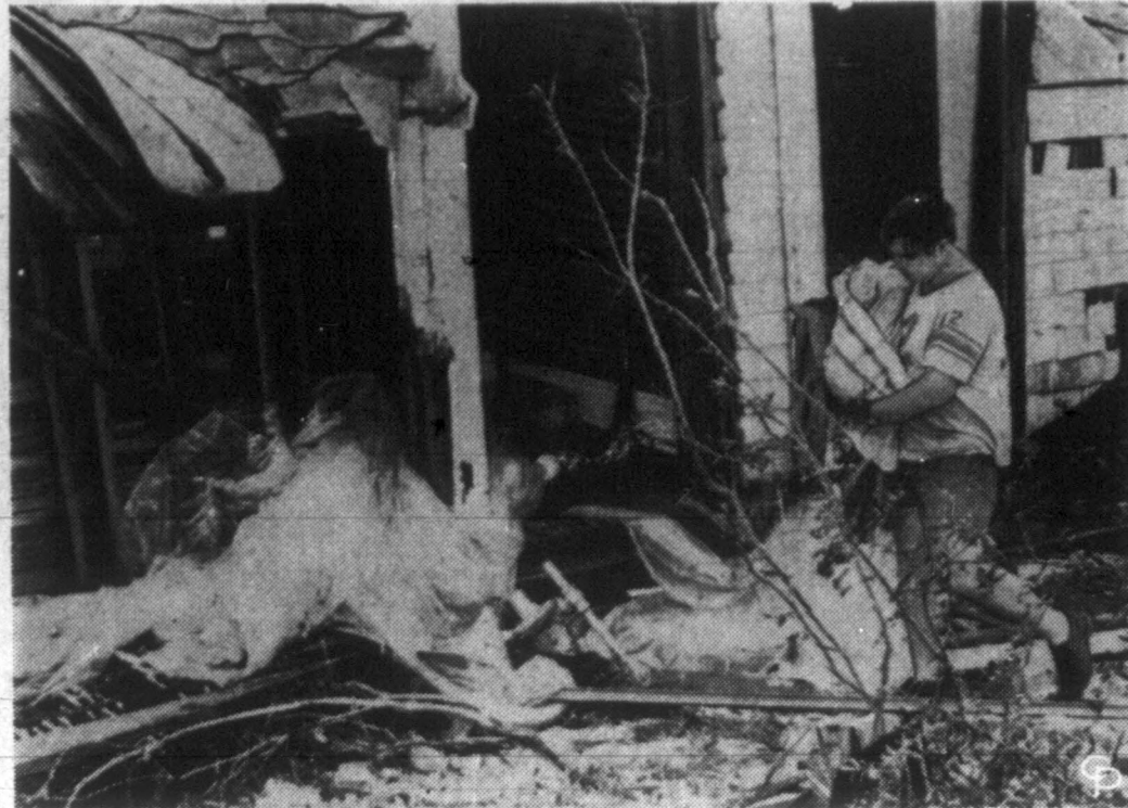
UPSTAIRS NOW DOWNSTAIRS—Robert L. Bradshaw, 17, removes belongings from his second-floor apartment which now is the ground floor in the wake of Hurricane Camille at Gulfport, Miss. The 190-mph wind took the ground floor right out from under.
